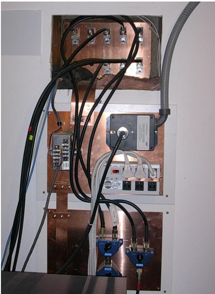
Inside view of antenna and cable entrance panel with protectors
